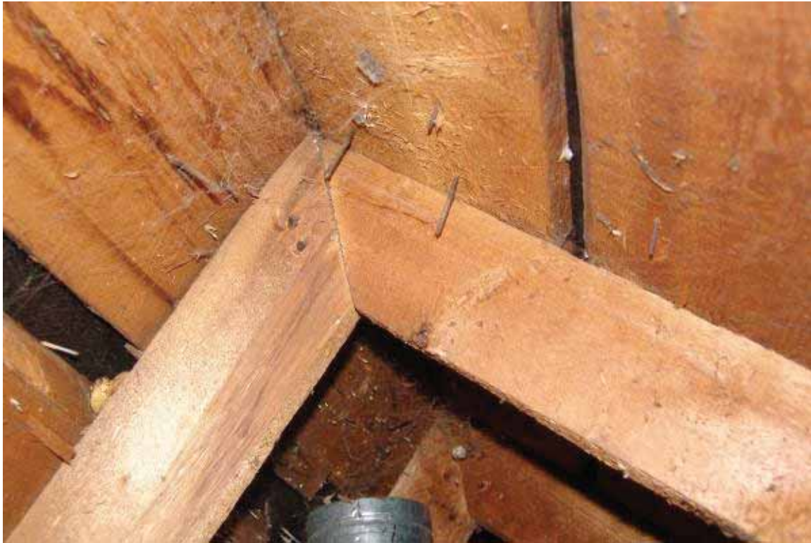
Photo 3.3-12: Ridge of the main building roof. Note the lack of a ridge board and the two toenails
