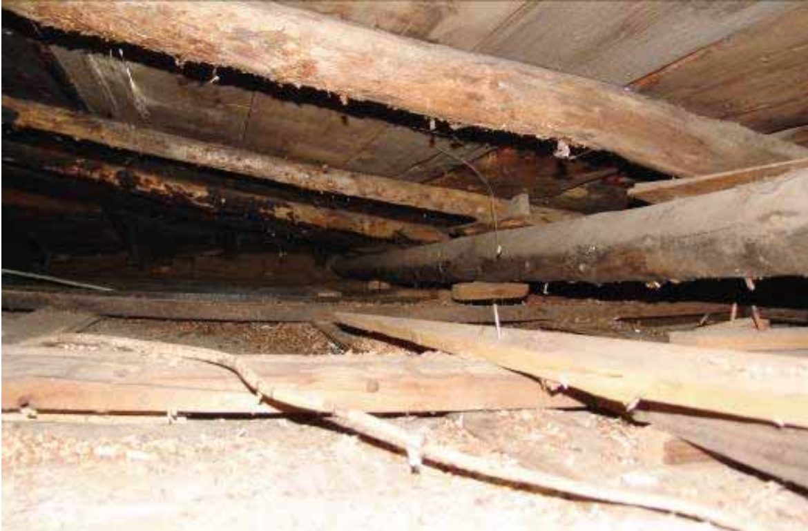
Photo 3.3-19: Dropped log purlin and rafters at the south lean-to addition above Room 3
