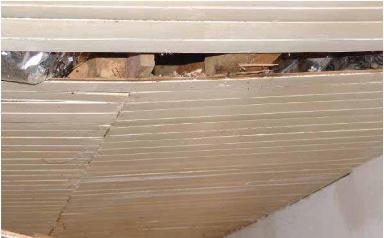
Photo 3.3-11: Seam in ceiling representing possible end of former load-bearing interior wall, Room 2. Discontinuous joist end visible at aperture in ceiling.
