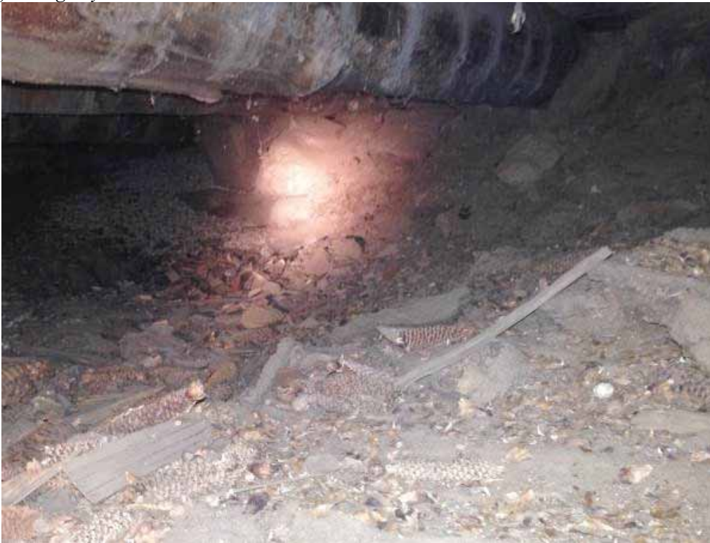
Photo 3.2-6: Loose stack of stones supporting the chimney above
