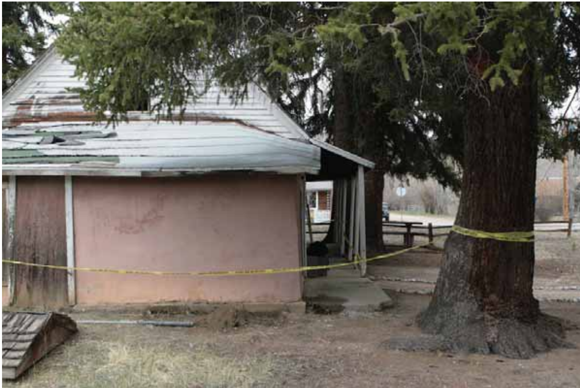
Photo 3.5-4 showing collapsing roof in south addition.
