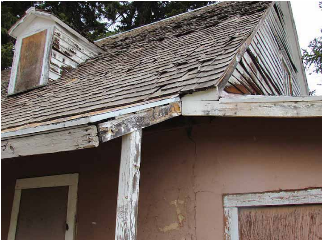
Photo 3.5-1. West side dormer, south side gable siding, west side fascia and roofing.
