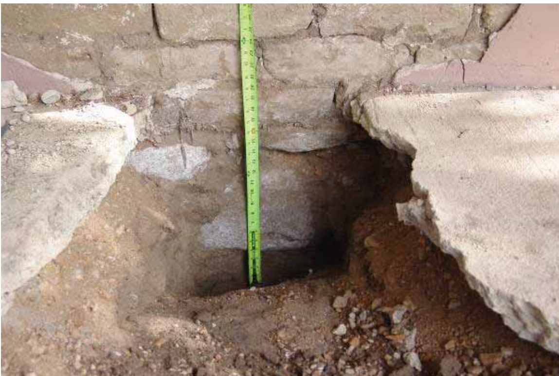
Photo 3.2-2: Depth of foundation as measured from exterior exploratory excavation along north elevation
