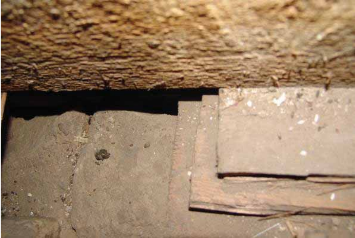
Photo 3.3-7: Second floor end joist bearing on wood shim stack over adobe wall
