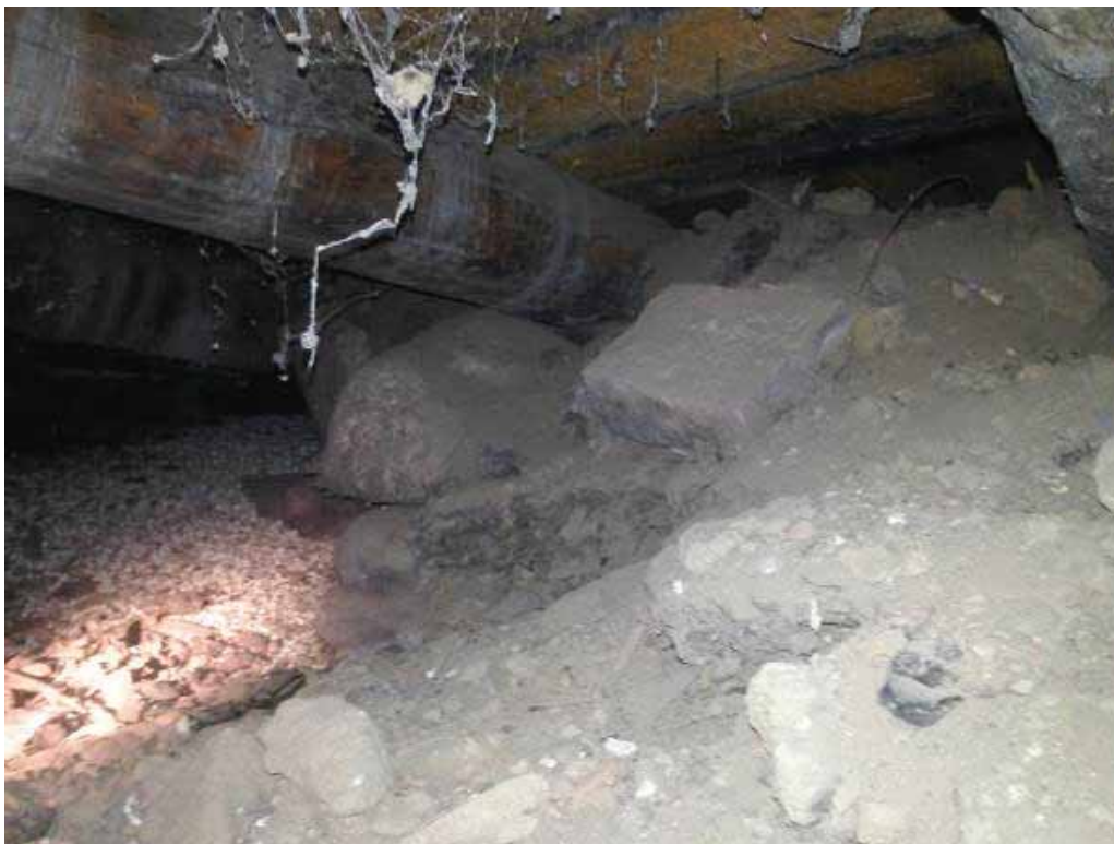
Photo 3.2-14: Rubble stone footing beneath chimney has spilled outward into the crawlspace
