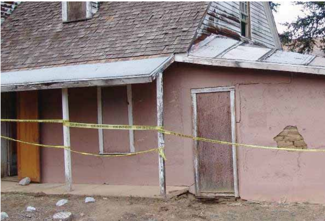
Photo 3.4-11: Stair step crack along west elevation. Crack originates at edge of slab where foundation discontinuity and rotation is suspected.
