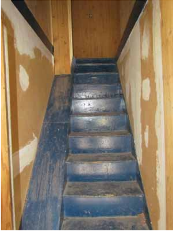
Photo 2-11. Looking up historic stair. Enclosure has been widened to accommodate furnace flue.
