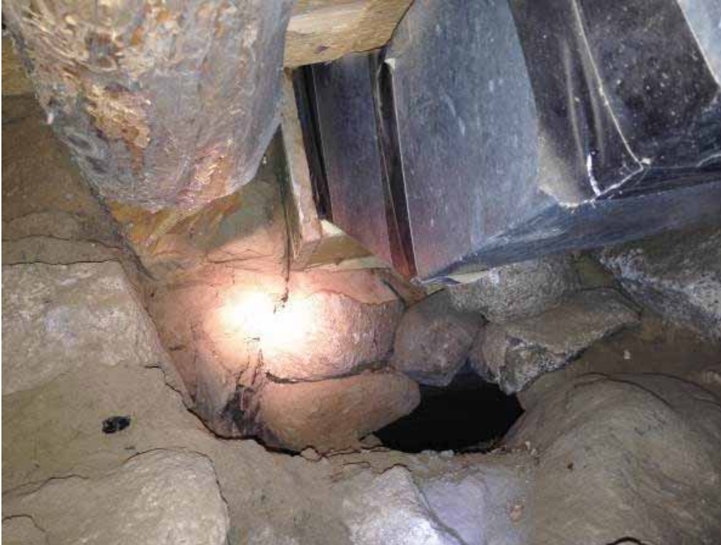
Photo 3.2-12: Inside face of stone foundation wall along south elevation of main building in south bay below Room 2. Note that opening made for duct has undermined the log floor joist.
