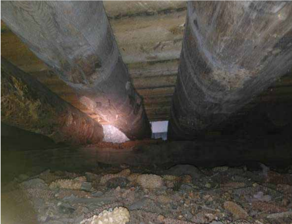
Photo 3.3-1: First floor log joists in the south bay of the main building looking north at log sill
