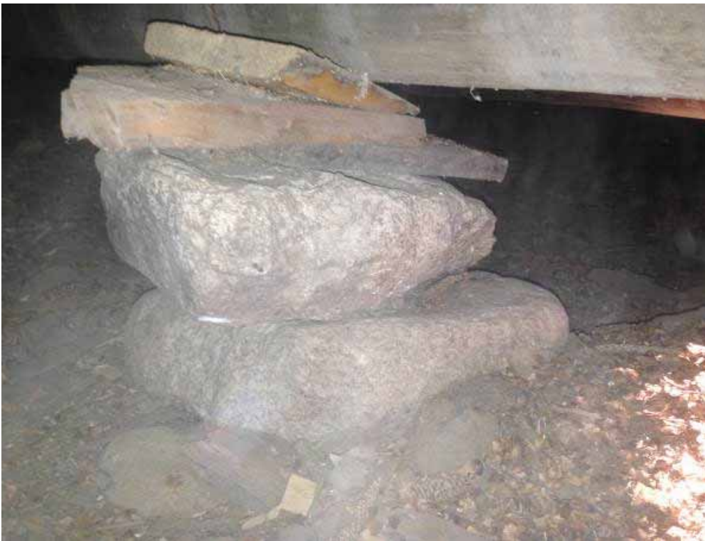
Photo 3.2-4: Singular stacked stone support at midspan of a log joist in the south bay
