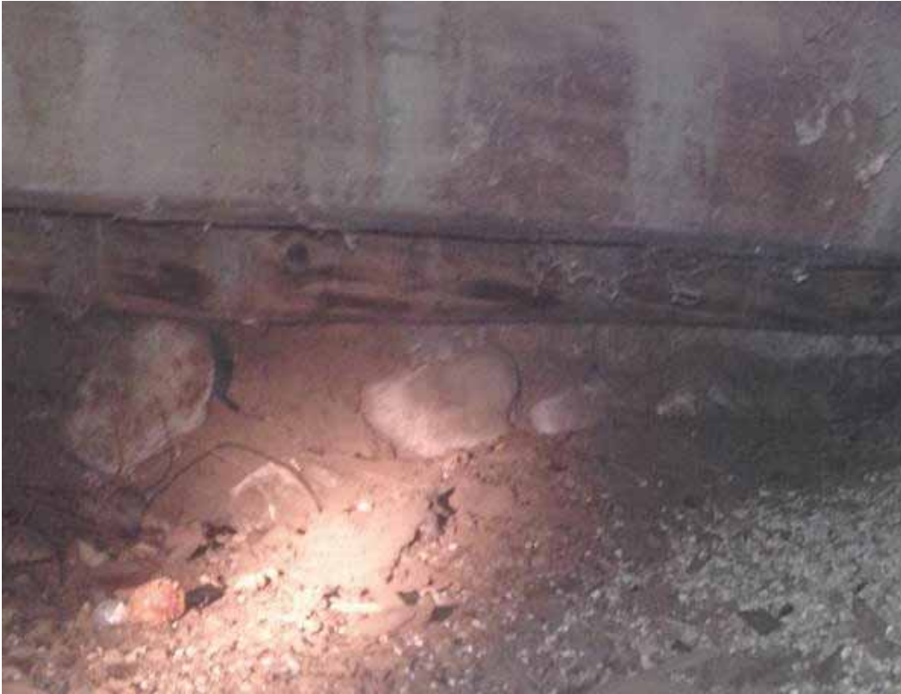
Photo 3.2-11: Inside face of stone foundation wall along east elevation of main building in south bay below Room 2
