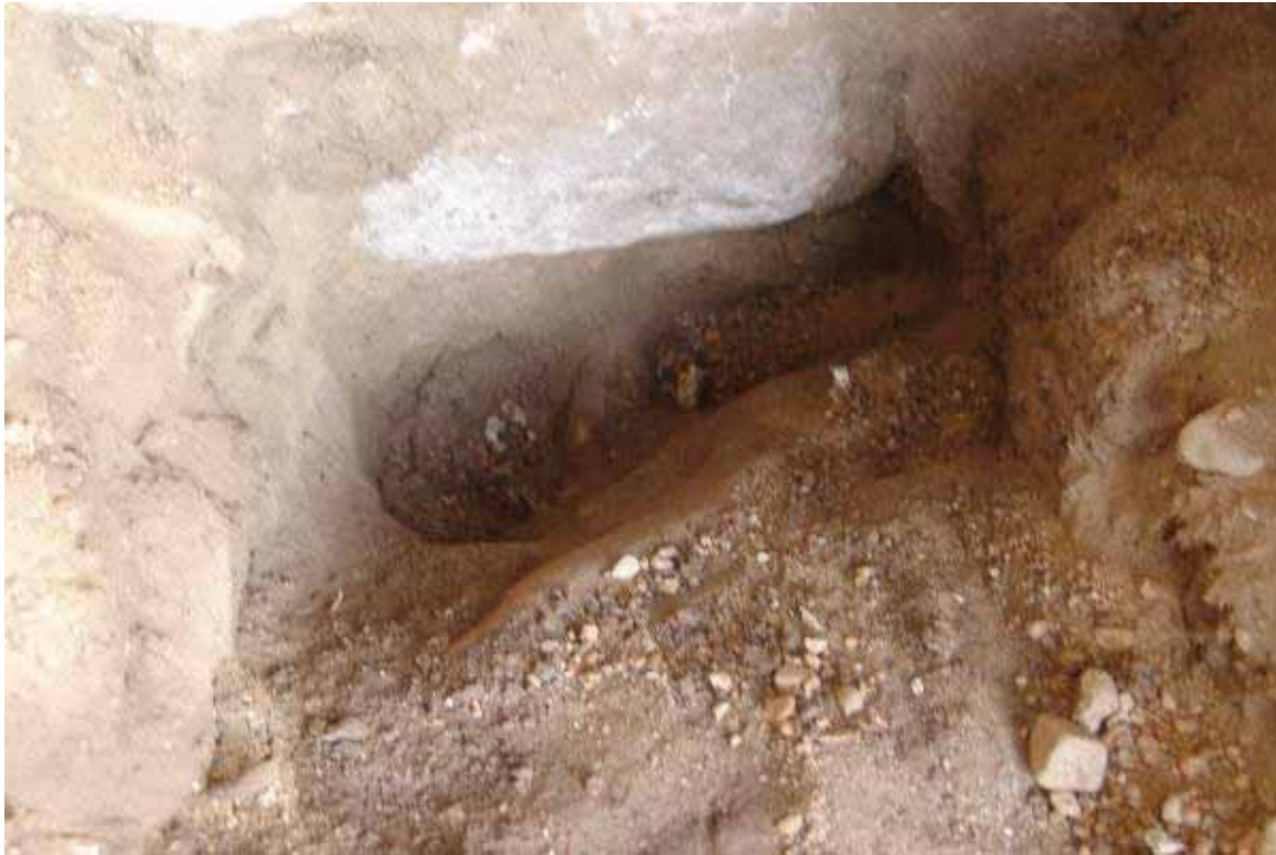
Photo 3.2-13: Base of foundation wall along north elevation. Note that tree root is oriented parallel to foundation wall and that it has not displaced the immediately adjacent stones.
