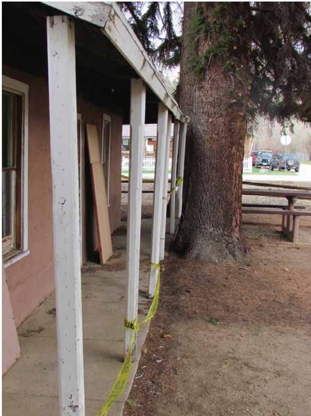
Photo 3.5-2 showing north porch roof deflection.
