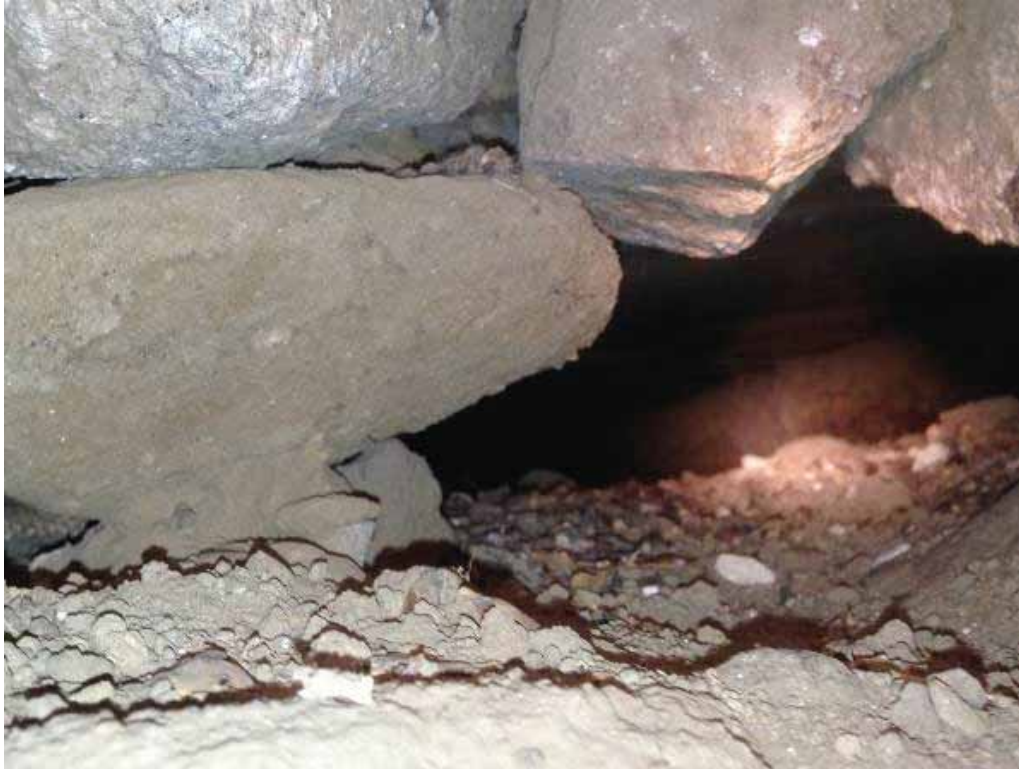
Photo 3.3-4: Log joist resting on or near crawlspace soils faintly visible in background beyond hole in foundation wall.
