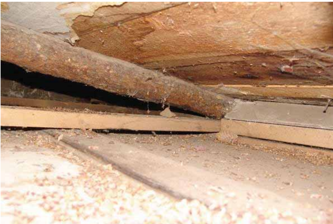
Photo 3.3-18: Rafters and ceiling joists at south wall of south lean-to addition above Room 3
