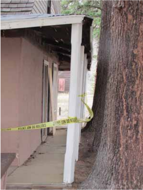
Photo 3.1-4. Looking west along north porch showing concrete porch slab, porch roof and spruce trees
