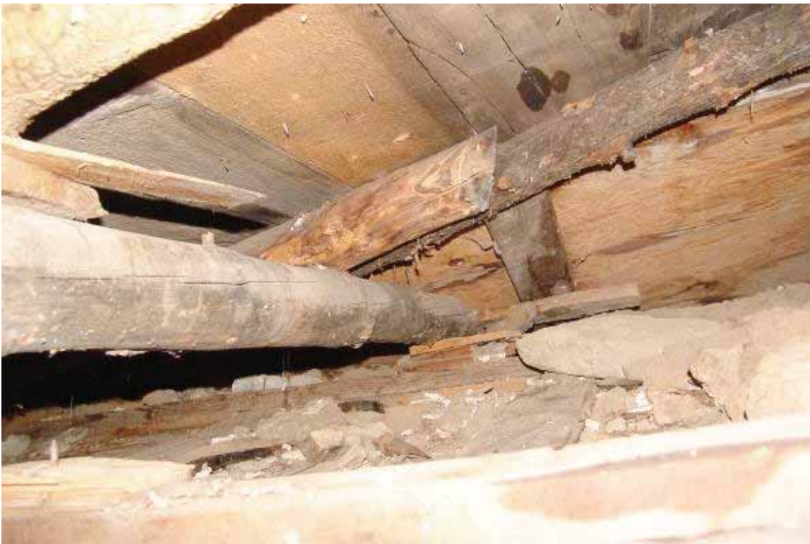
Photo 3.3-20: Log hip and flat 2x4 rafter at south lean-to addition hip above Room 3
