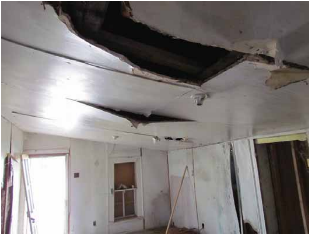
Photo 3.5-3 showing collapsing roof/ceiling in south addition. Room 3, interior.
