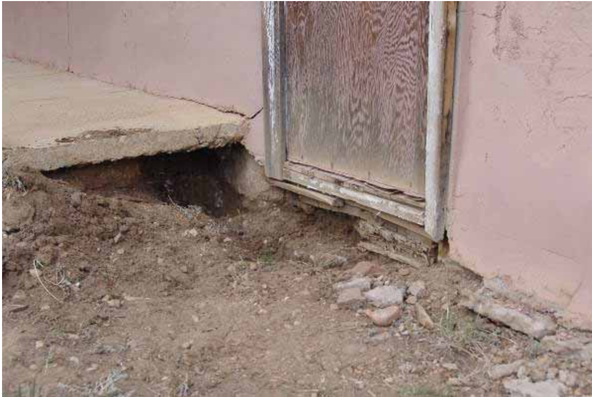
Photo 3.2-9: West elevation of south addition. Note multiple layers of floor sheathing and threshold elevation relative to apron slab
