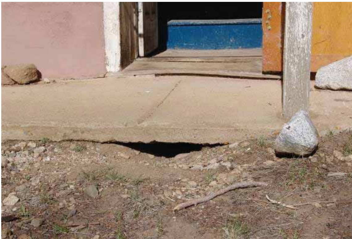
Photo 3.2-2: Burrow hole beneath exterior concrete sidewalk, west side
