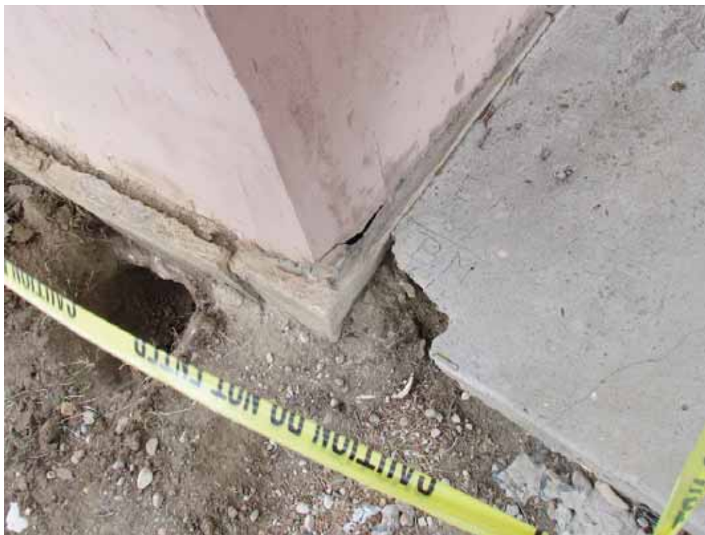
Photo 3.2-1: Exterior sidewalk damage and burrow hole at southeast corner
