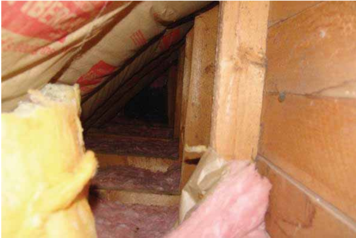
Photo 3.3-9: Dead space along east and west sides of second floor. Note cripple studs supporting rafters and unsheathed second floor rafters
