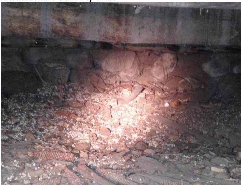
Photo 3.2-10: Inside face of stone foundation wall along west elevation of main building in south bay
