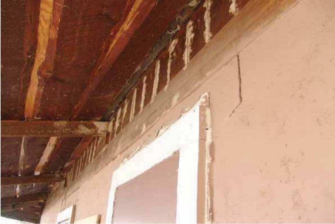
Photo 3.4-10: Cracks in stucco at door and window head corners along north elevation
