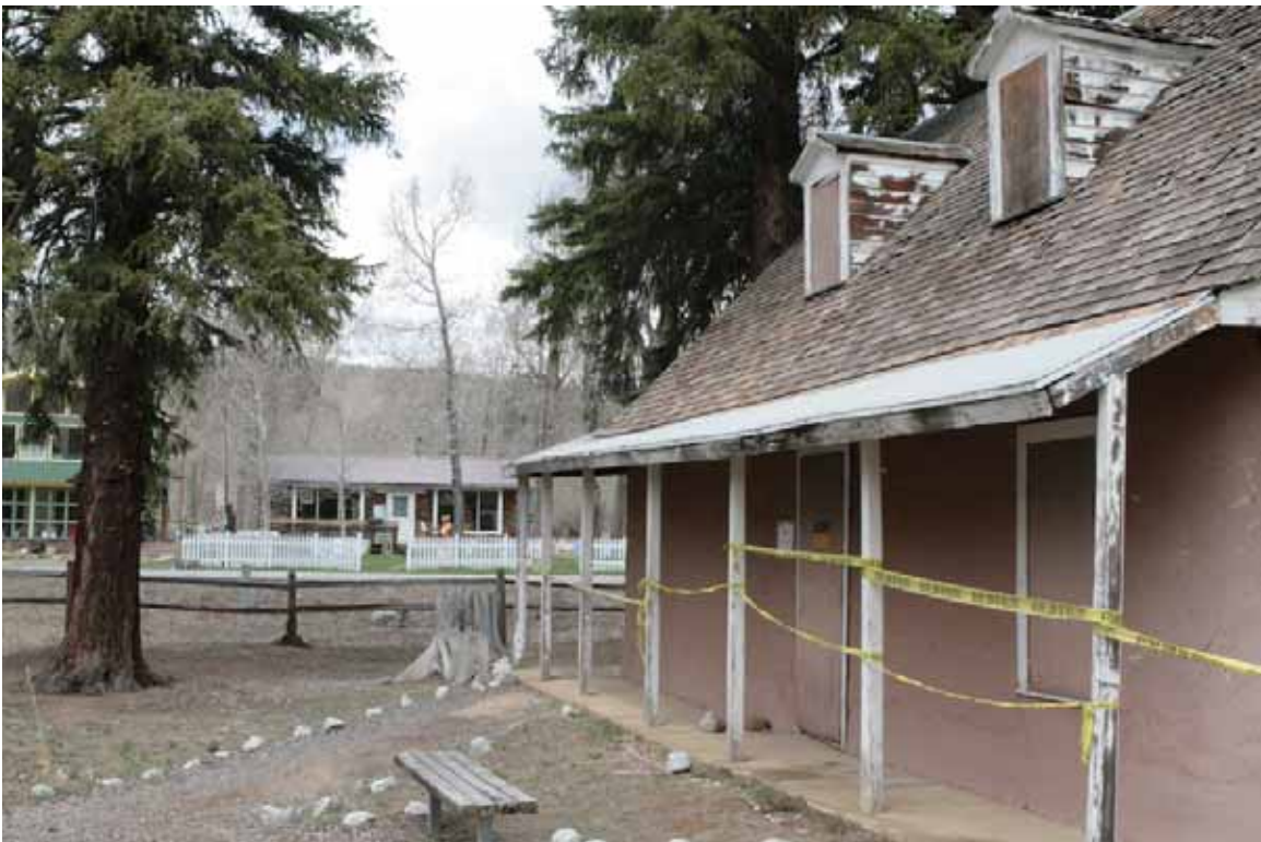
Photo 3.1-5. Looking north along west porch showing concrete porch slab, porch roof, footpath with stone edging
