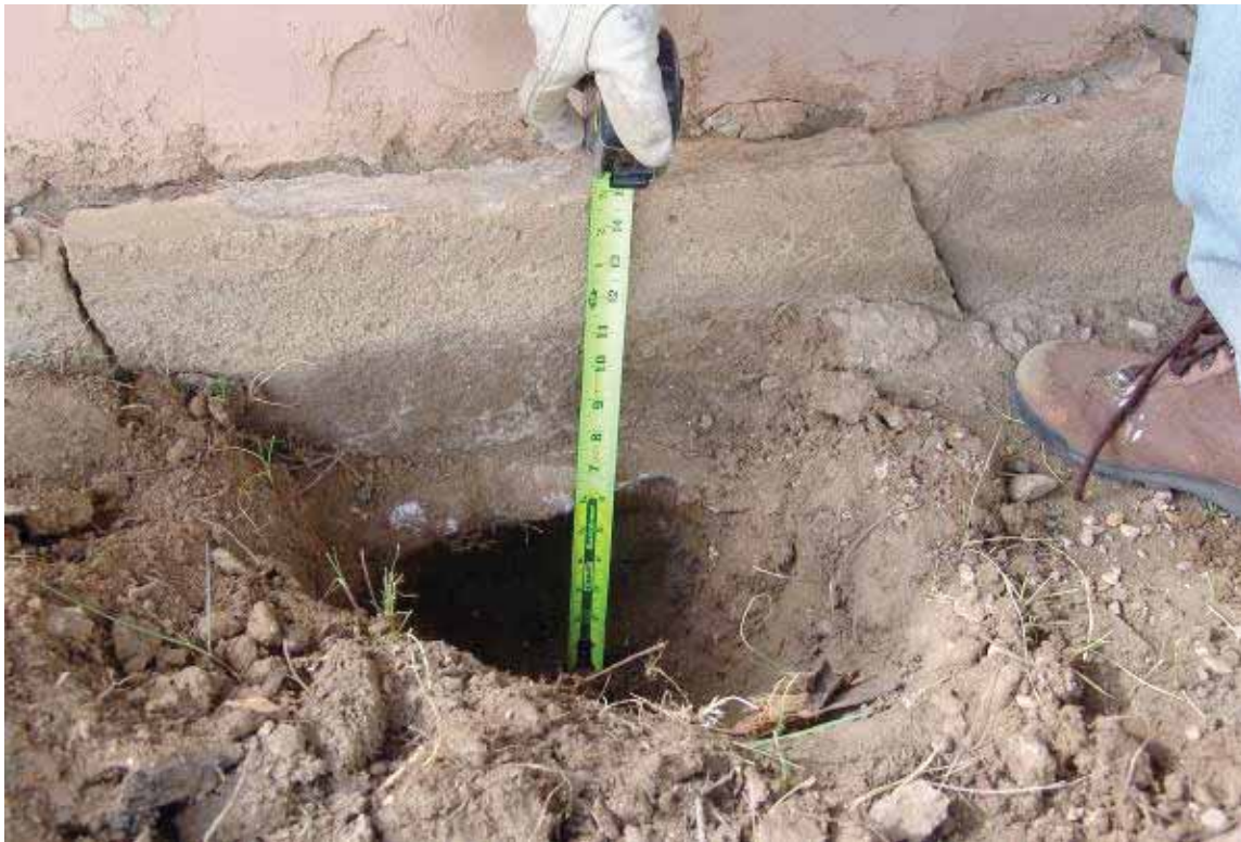
Photo 3.2-7: Depth of foundation as measured from exterior exploratory excavation along south elevation of lean-to addition
