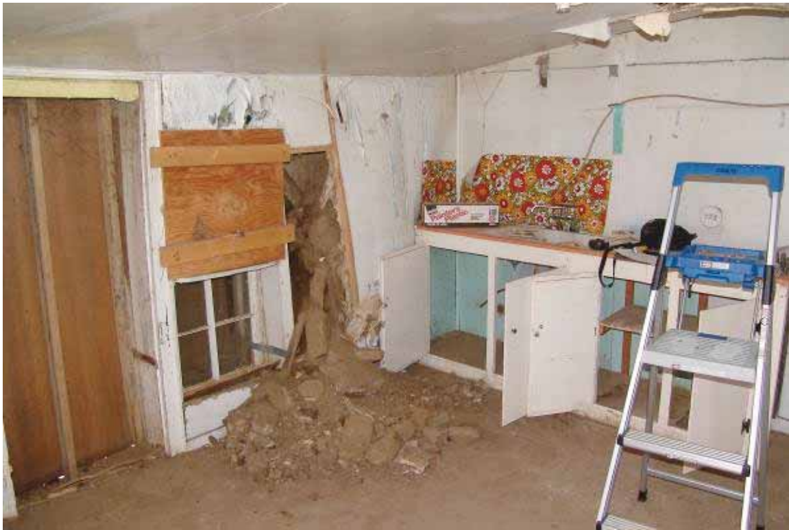
Photo 3.4-12: Collapsed south wall of lean-to addition (inside Room 3)
