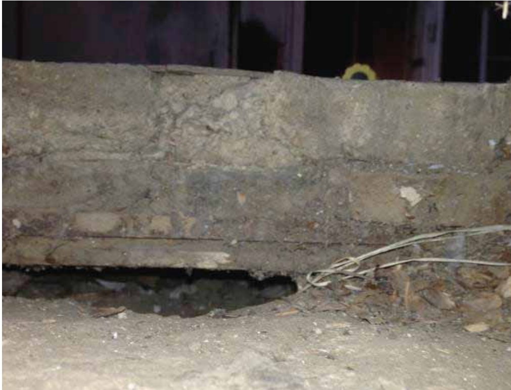
Photo 3.3-3: Cross section of floor sheathing and finishes in lean-to addition under Room 3. Note upper layer of concrete.
