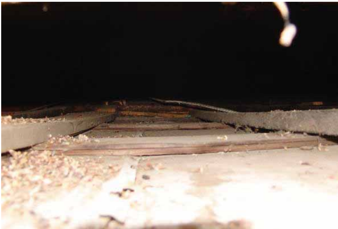
Photo 3.3-10: Lean-to addition ceiling joists and furring strips. Rafters are concealed in shadow
